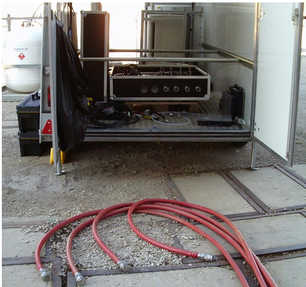
Figure 1.1 NPL CRF facility.
